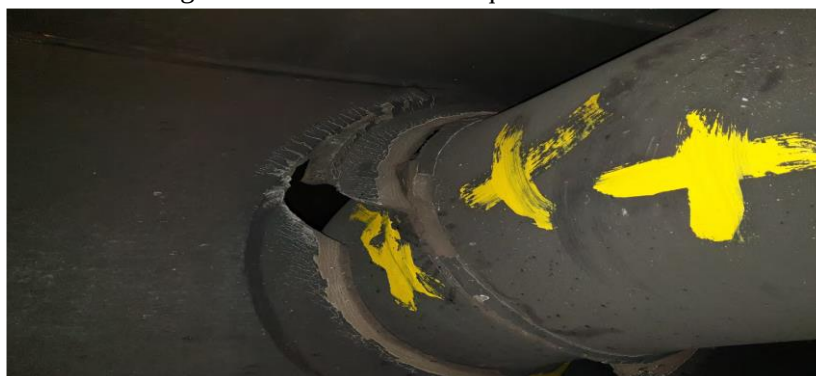
Fig.3. Bulkhead penetration of Marpol Line
