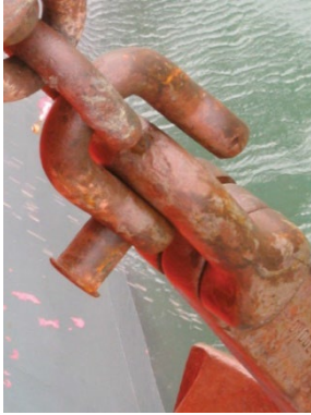
Pic. 3 D-link bolt almost loss due to missing securing pin
